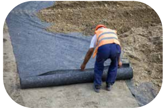
Worker laying geotextile in preparation for new building used for separation and reinforcement
